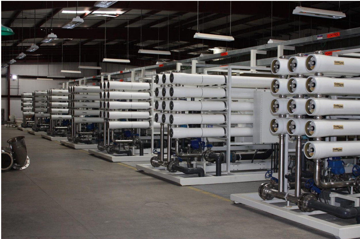
Figure 3-5: RO Equipment in a Pre-engineered Metal Building
