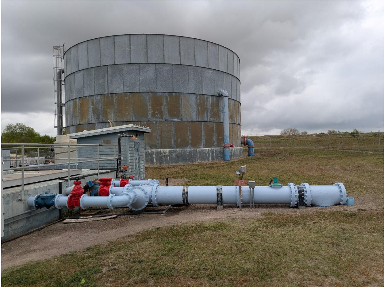
Figure 3-1: George P. Morrill WTP
