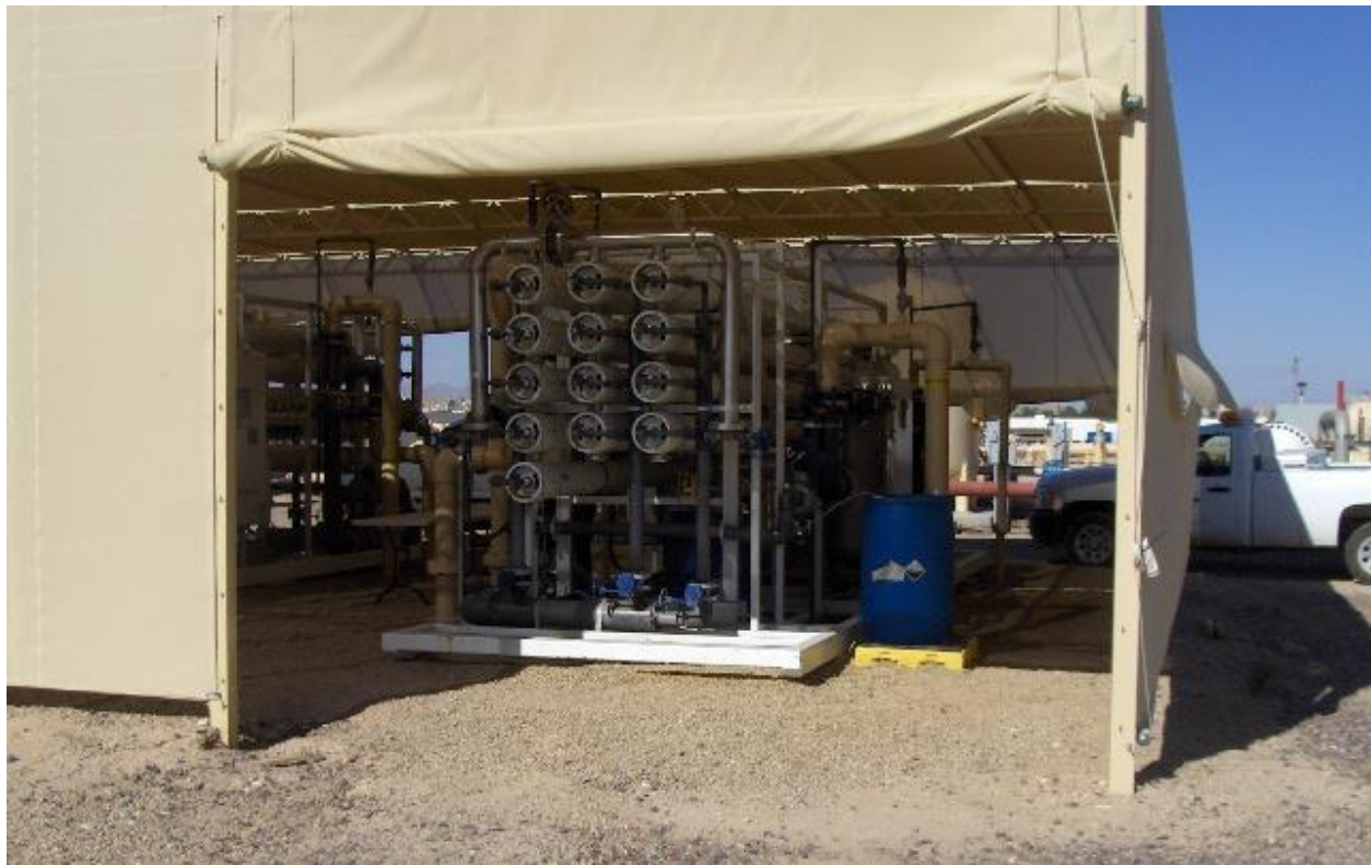
Figure 3-2: Well Head RO System with Equipment Under Canopy (Goodyear, AZ)
